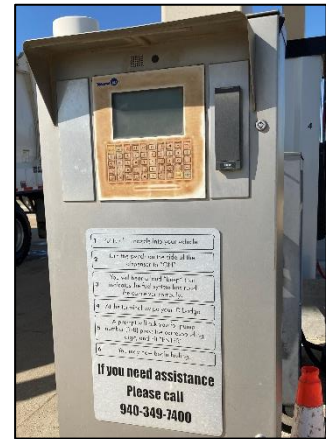
Picture 2: Manual Entry Station
